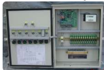
* RABH Control panel
